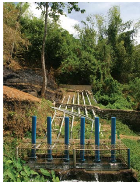
Air chambers and delivery pipes for six ram pumps that are used in parallel to supply more water at this site 'I'll like the third shot of this the best'
