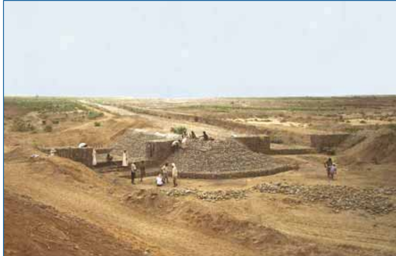
FIGURE 4.23 Gabion flow bifurcation structure in Eritrea
