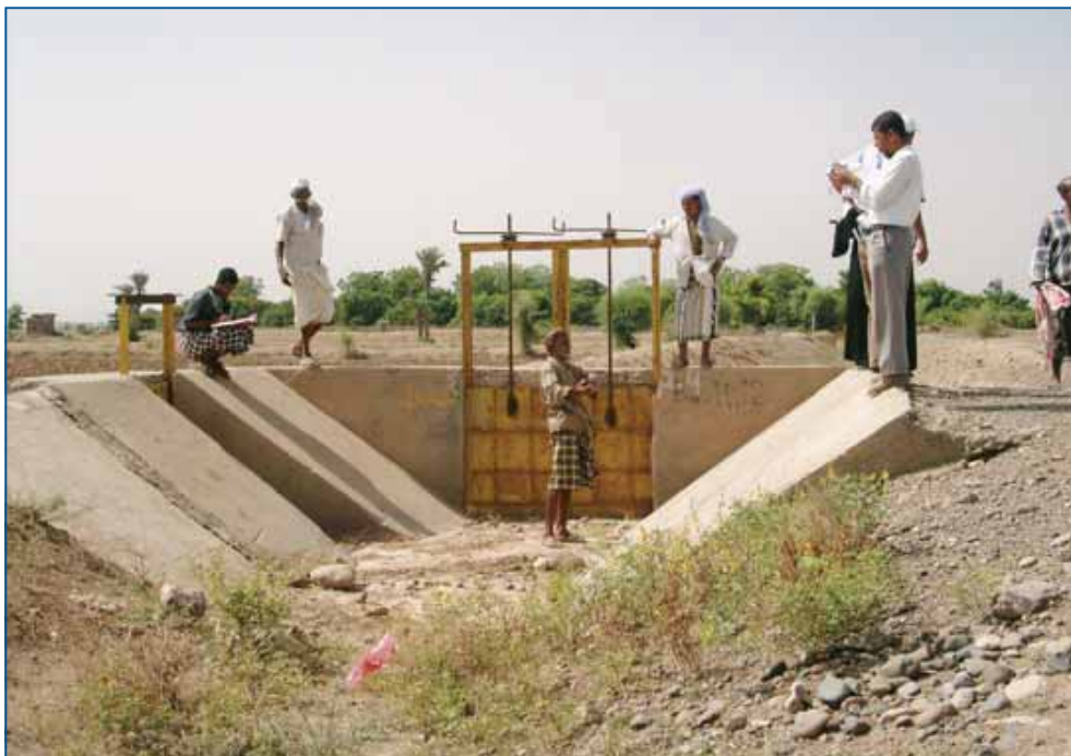
FIGURE 4.22 Gated combined check/drop structure in Yemen
