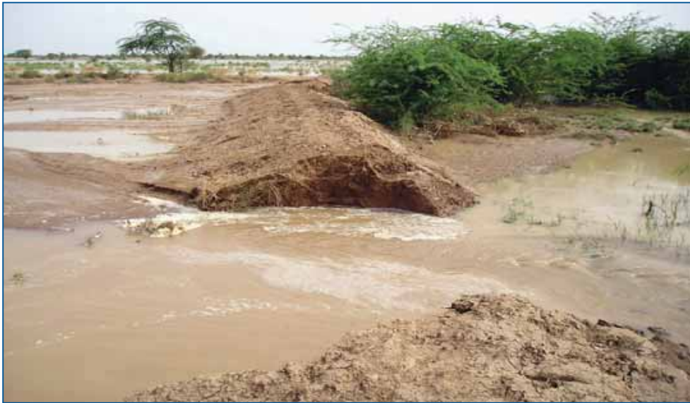
FIGURE 4.6 A breach in a deflecting spur in Eritrea
