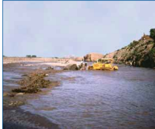
FIGURE 8.2 Bulldozer repairing a traditional diversion spur during a flood recession. Wadi Rima, Yemen.
