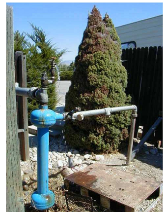
A typical wellhead.
