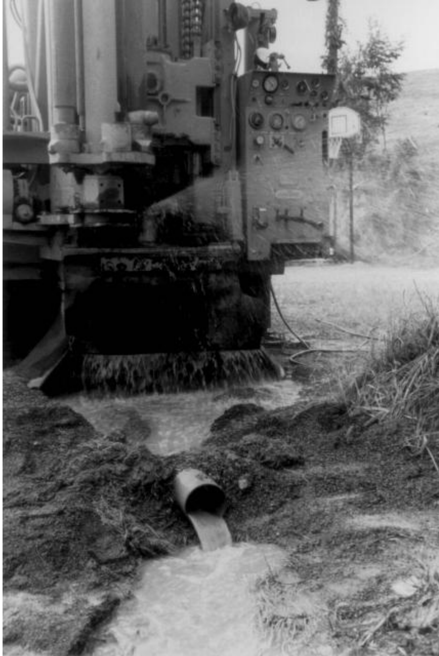
Photo shows the water flow from a newly drilled well.
