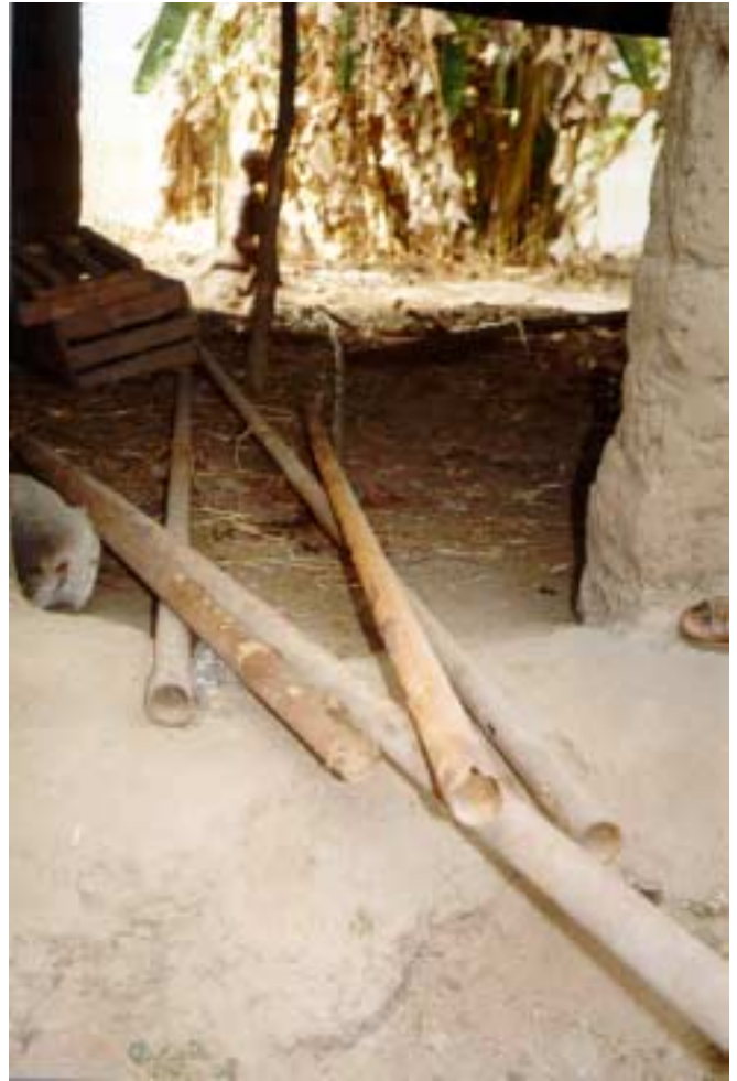
Figure 7.2 Highly corroded rising main from a borehole with TDS greater than 3000 mg/l. New rising main corroded within one year.
