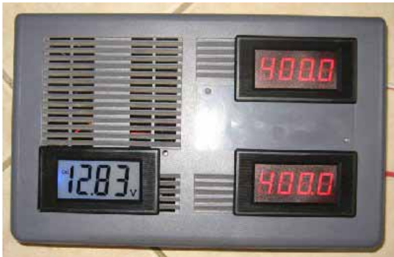
Digital control panel
