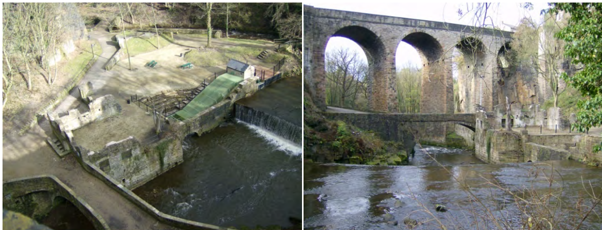
Figure 2. (Left) plan view photo of the RAS at New Mills and (right) a photo looking across the top of the weir to the angled transect (left-hand arch) and same axis (second arch in from right) NB: the bridge is indicative of the stone cliff heights around the site.
