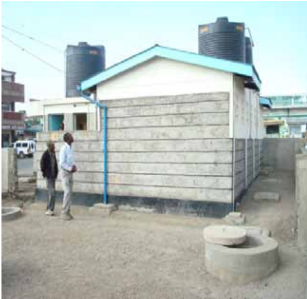
Combined public toilet , bathrooms, digester, water kiosk - Naivasha
