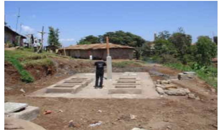
Bio-digester & baffle reactor - schools and prisons
