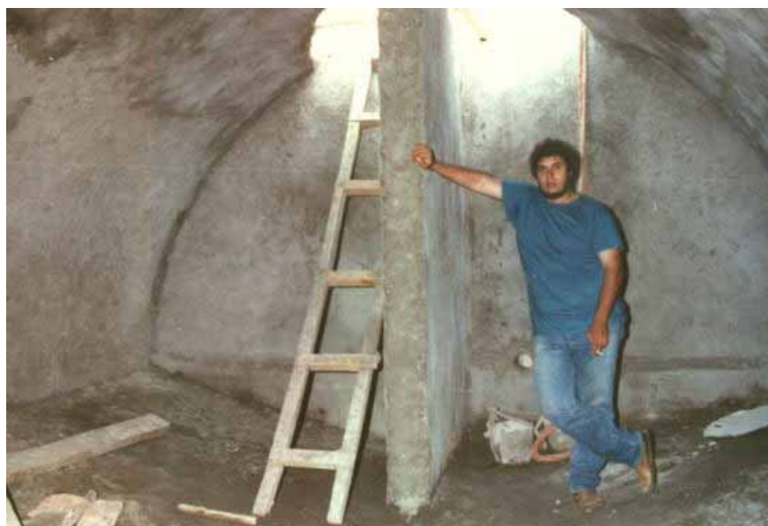
View in a canal digester, Burundi
