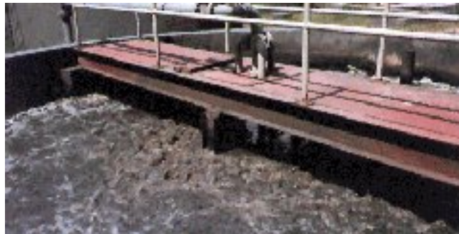
Figure 3.1 Photo of an aerobic digester 3
