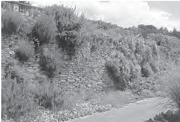
Plate 130 This classic example of a planted drystone retaining wall is at the restored Jekyll and Lutyens garden at Hestercombe in Somerset, UK.
