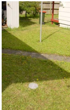
Photo 1 Nominal Soakhole: Installed beneath a grassed area--This example has an inspection well topped off with an alloy toby box.
