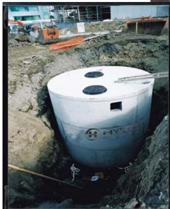
Photo 7 Sand-filter 1 Large sand-filter on a commercial site (photo supplied by Hynds)
