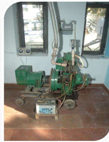
Biogas used for electricity generation
