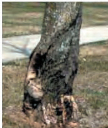
Figure 3.131. High risk of failure: When canker affects 40 percent or more of the tree's circumference.
