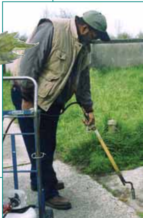
Torches work on weeds in cracks or gravel
