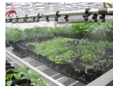
Figure 12: Boom irrigation system
