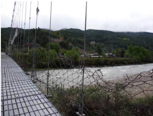
A badly maintained bridge
