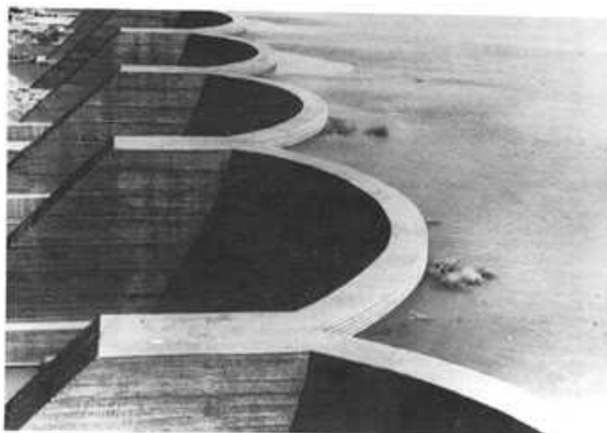
Plate 6.8 A large sediment trapping dam, Republic of South Africa, using an ingenious method of construction which reduces the amount of concrete required. The shuttering for the arches is made from corrugated roofing iron
