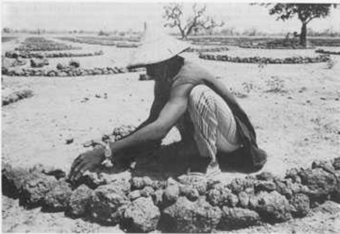
Plate 7.6 Building the low stone wall with lumps of laterite, Burkina Faso (OXFAM)
