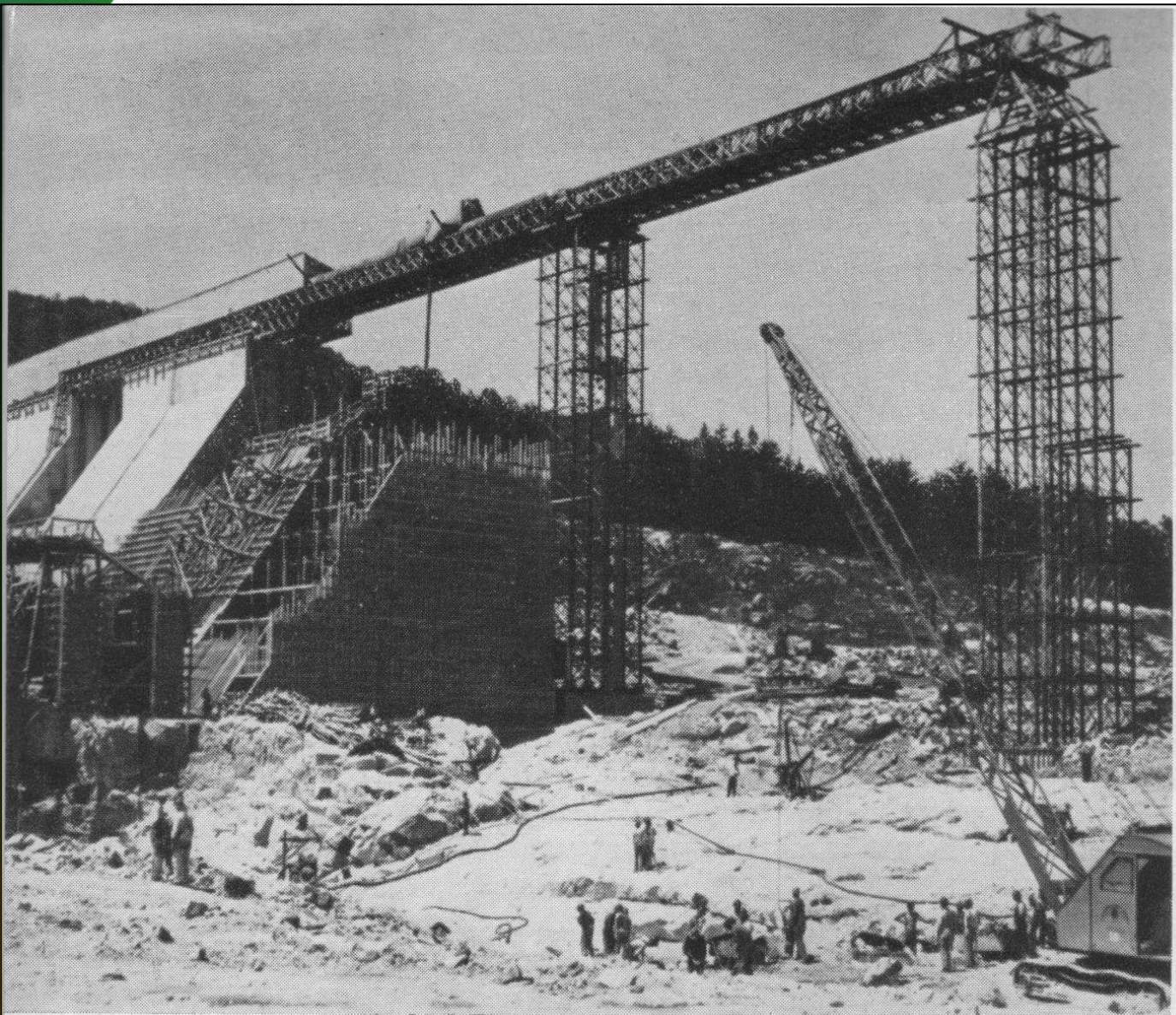
Bailey Towers and Trestle Supports for Conveyor at Des Joachims Dam
