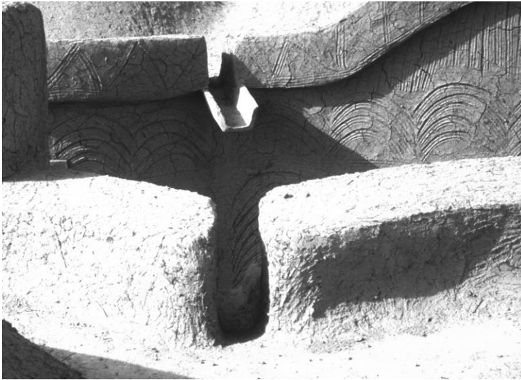
Figure 4: Violent storms require good water management using graded slopes and open gutters.
