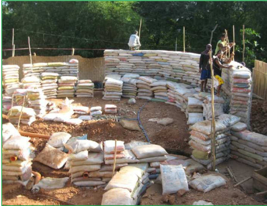
Sandbag construction in the Philippines? Long sandbags add stability, but using barbed wire between layers of shorter sandbags, is also fine. It takes much longer to fill the long bags than the short ones. Photo by SCDLR8899 www.flickr.com
