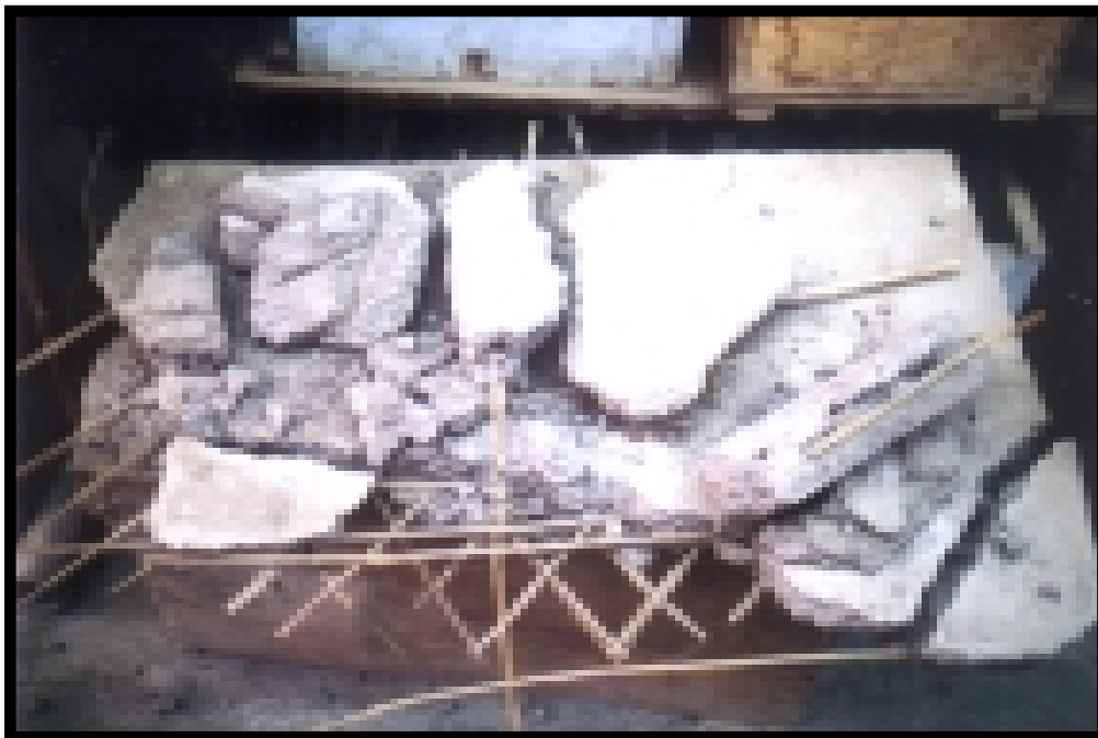
Fig. 81: A failed example of bamboo-reinforced concrete
