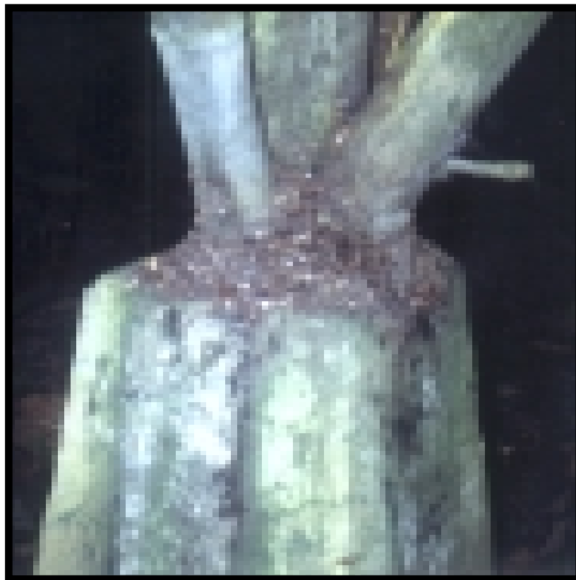
Fig. 36: Concrete foundation for a bamboo building, but the bamboo gets wet enough to invite fungal and insect attacks
