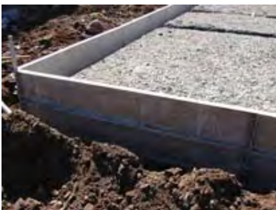
A formwork for foundation, panels mounted on top of each other, side by side and at the edge
