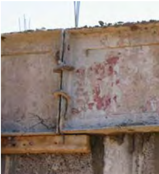
A formwork for a slab, fixed by additional wires bound to the reinforcement of the slab
