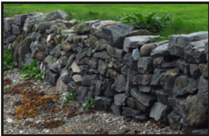
An exceptionally poor newly-built retaining wall. This wall displays all the features of a wall that should not be accepted.
