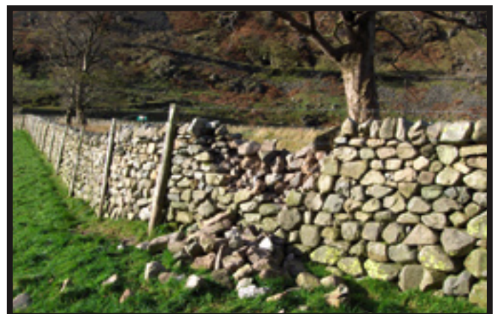
The only damage in this wall is next to the tree!
