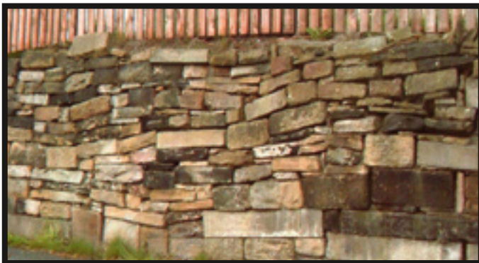
An extreme case of sloping stones. This is a very poorly built wall with lots of defects, despite the exceptionally level bedded and regular stone. (Photo: Dry Stone Walling Techniques and Traditions 2004)
