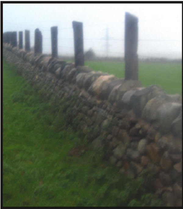
A wall with slate and wire fence above. In this case because the wall was low and narrow, the cope and slates are mortared.
