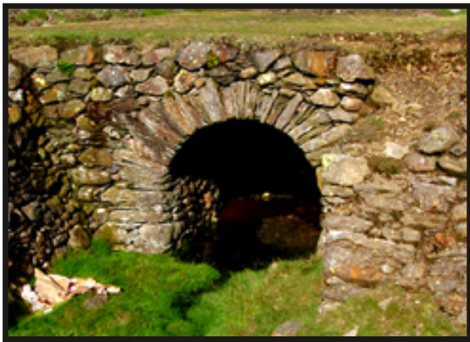
A dry stone arched culvert at the copper mine ruins in Coniston.
