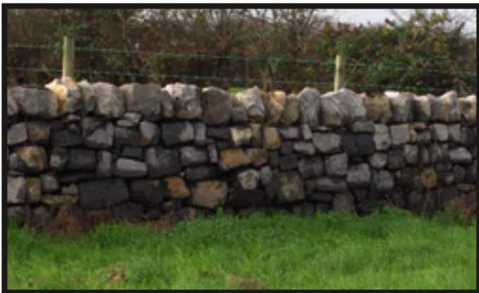
This new roadside wall is full of running joints.
