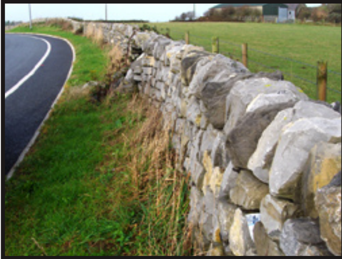
A five year old roadside wall in Anglesey Wales. The wall was very poorly built and sections have already fallen, as shown in this picture.
