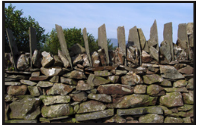
An unusual buck and doe cope that uses old roofing slate which makes an excellent deterrent to keep sheep from attempting to jump the wall.
