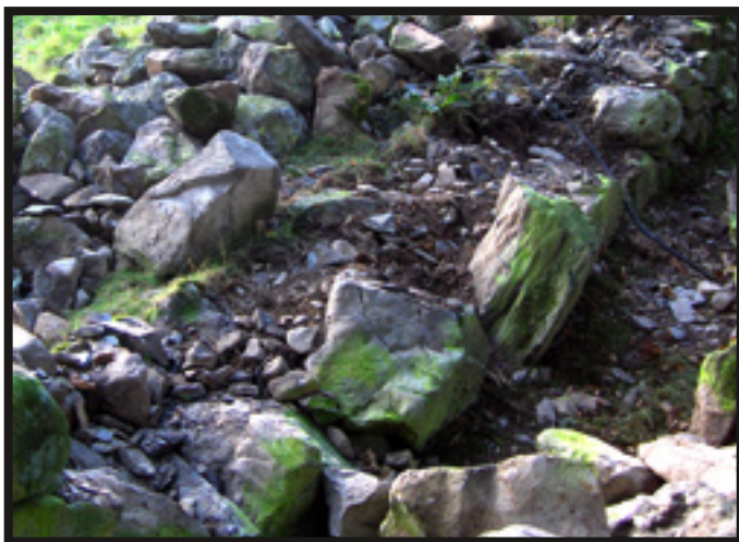
Existing footings in need of resetting. The large stone near the center has a top that slopes steeply outward. The stone behind it was set on its edge and is now leaning outside of the plane of the wall.
