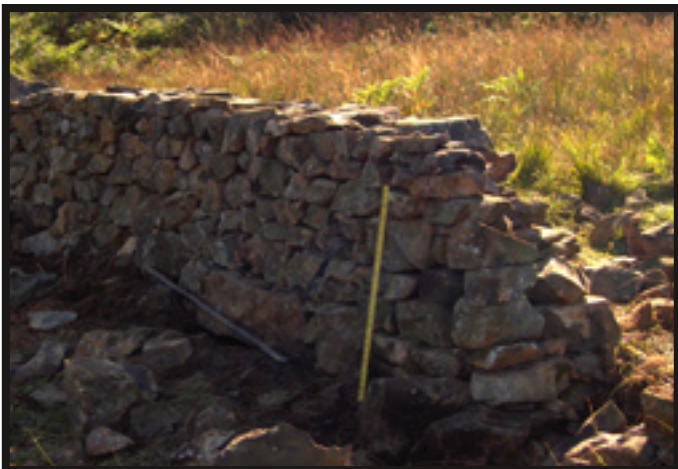
A wall being built of Silurian Slate, which is very irregular and difficult to build with.
