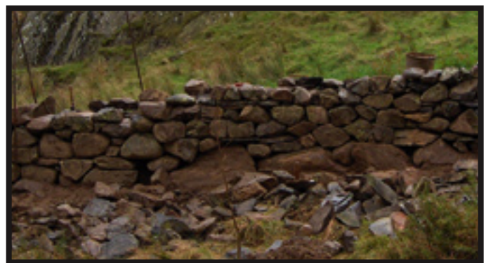
A wall being built using unusually large footings. These footings were irregularly shaped, and too heavy to move easily, so getting a perfect fit was impossible.
