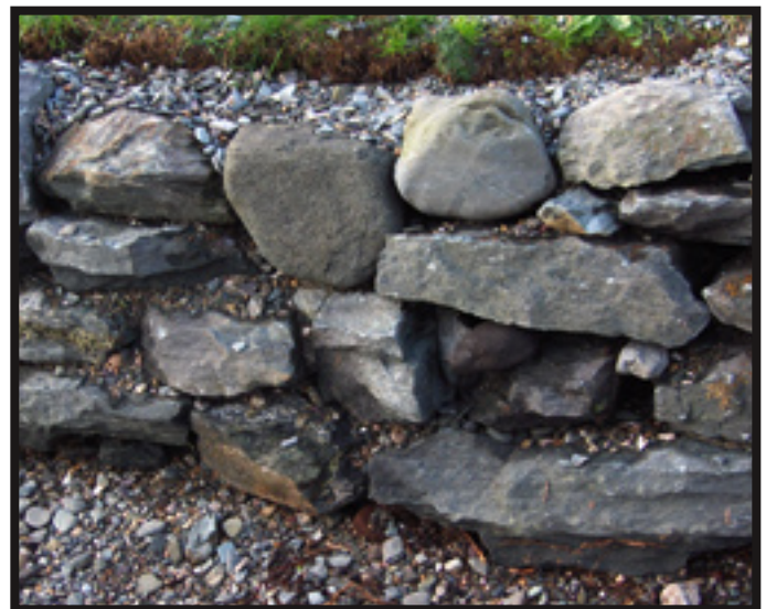
This retaining wall has been filled with gravel, and has many other problems as well. Walling such as this should never be accepted.
