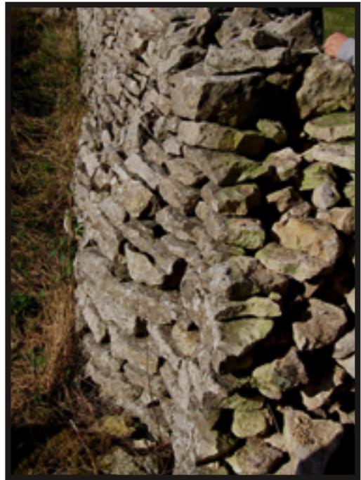
This Costwold wall was bulging dramatically...
