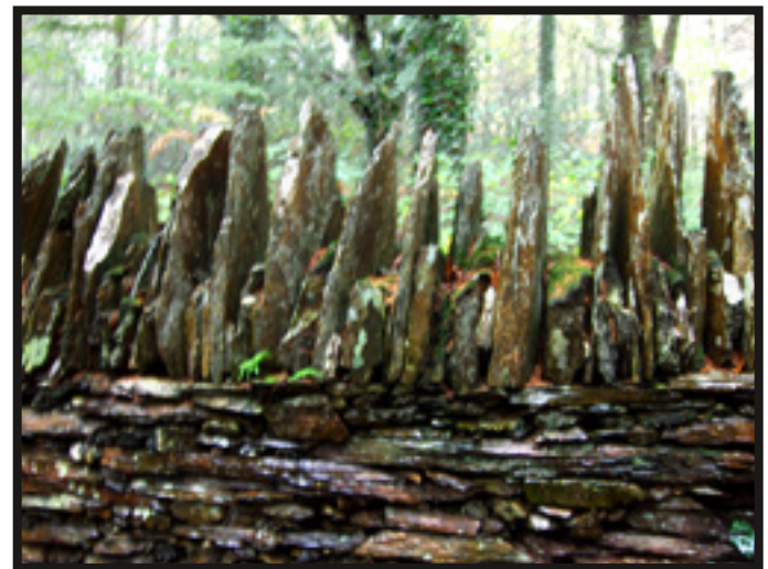
This unusually tall cope adds about 20" to the height of the wall.
