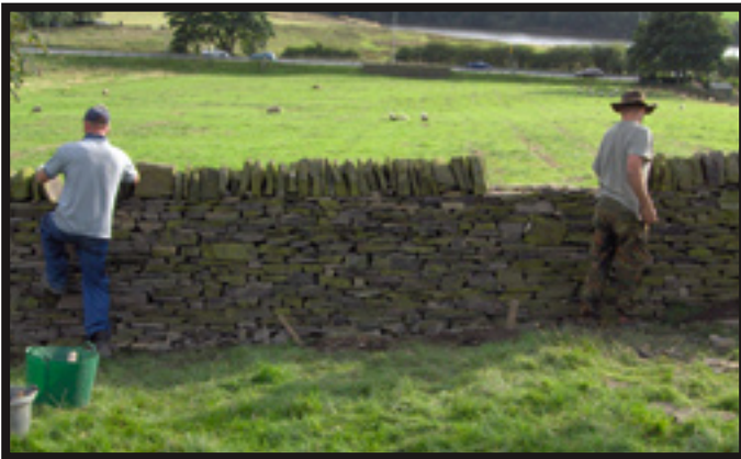
A nearly finished Initial level test wall. My section is in the center.
