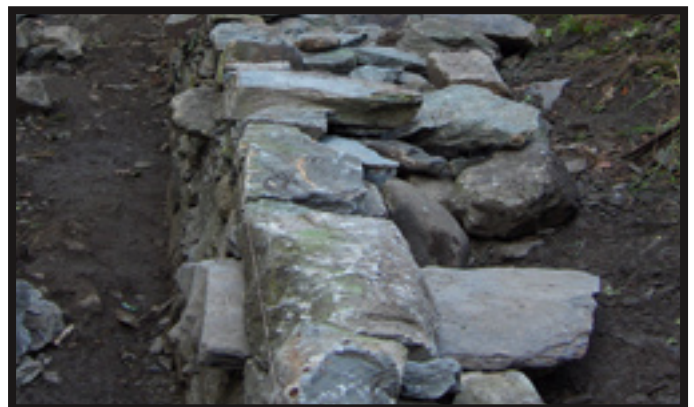
Placement of a “through” stone in a single retaining wall. In this case the throughs protrude from the wall face as is common in freestanding walls.
