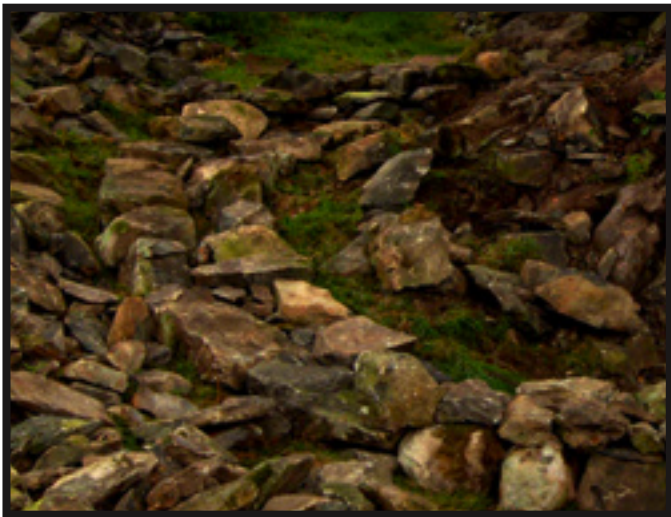
Footings set on grass for a new section of curved feild wall.
