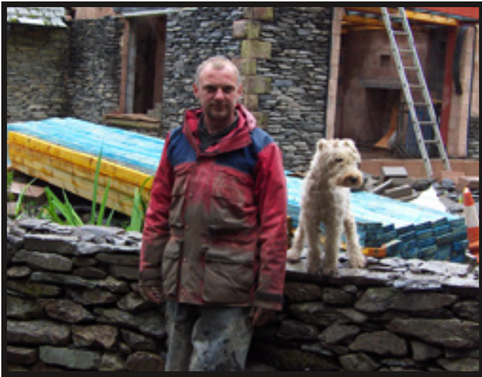
Andy, with his dog Tod in front of a wall being built.
