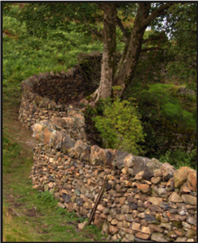
The solution was to build the wall around the tree, resulting in this rather curvy wall.
