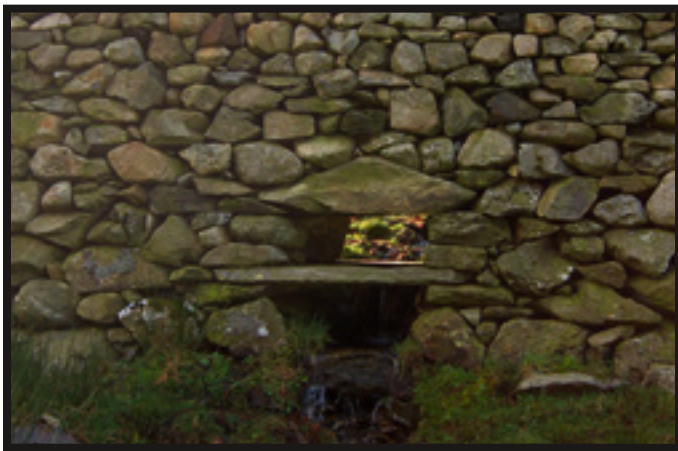
A large water drain , with a piece of slate across the middle to keep sheep from passing through.
