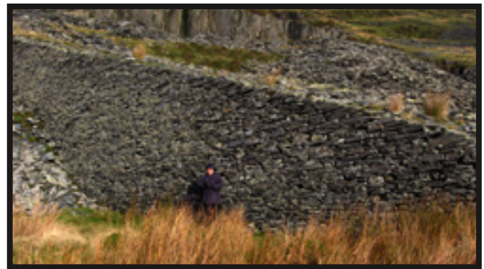
A tall retaining wall in an abandoned North Welsh slate quarry. This wall is one side of an incline ramp used to remove slate from the quarry. Note the scale figure at the center
