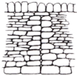
A wall double wall end. When on level ground such as this, it usually indicates a change in ownership of the wall. (Image: Brooks, 1999)
