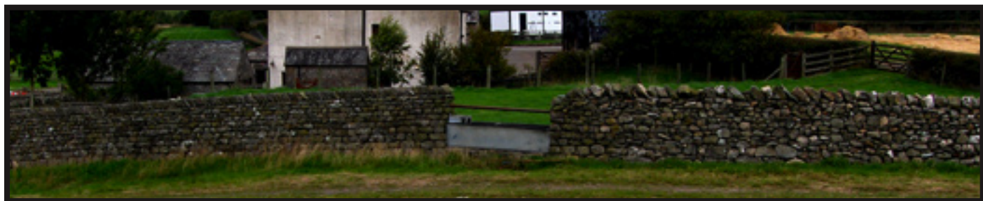
Coursed vs. Random. The wall on the left is built in rigid courses. The wall on the right is build randomly. Both walls are built with the same type of stone.
