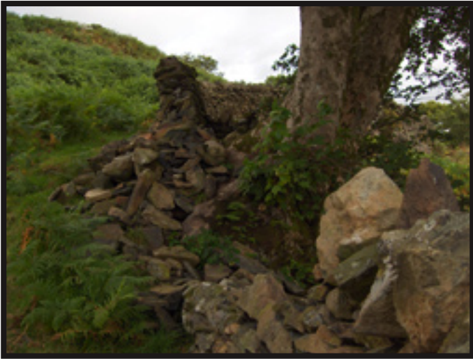
This wall was completely knocked over due to the tree roots flexing in a wind storm.
