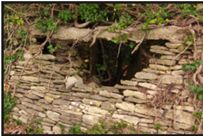
A wall that has fallen from under its mortar cope.
