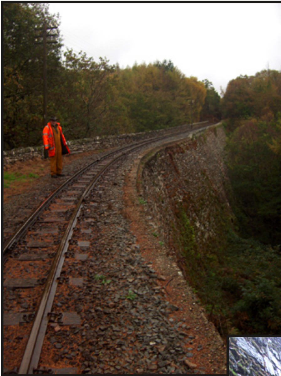
Looking along the wall from near the lower end. Much of the wall is now blocked from view by trees.
