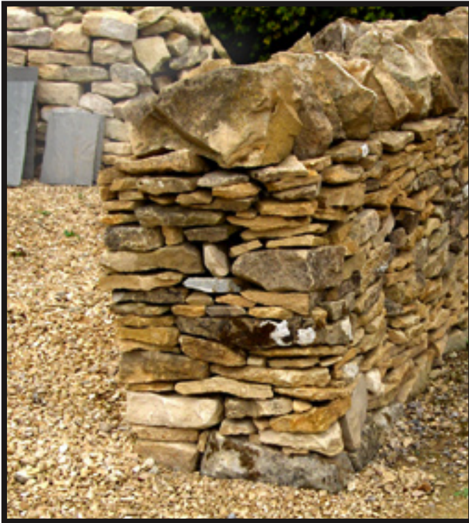
A very poorly built wall end. The sides are not tied together and the end is not tied back into the wall.
