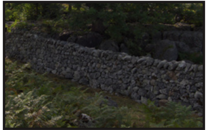
A wall built by Jerry and Vanessa with minimal use of string lines.
