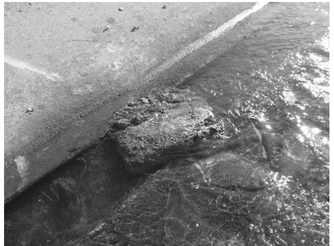
FIGURE 6: DESTRUCTION DE LA LONGRINE
