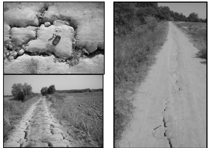
FIGURE 9: FISSURES DE DESSICCATION (SALMI ISL 2004)
