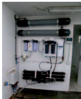
Figure 26. View of the MORENA SWRO unit.
