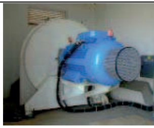
Figure 5. 100 kVA Synchronous machine coupled to flywheel.
