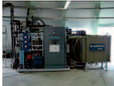
Figure 8. EDR desalination plant.
