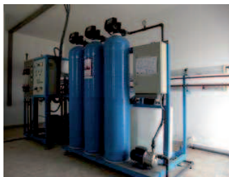
Figure 21. RO unit installed in Morocco.
