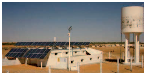
Figure 19. General view of the PV-RO system in the village of Ksar Ghilène (Tunisia).
