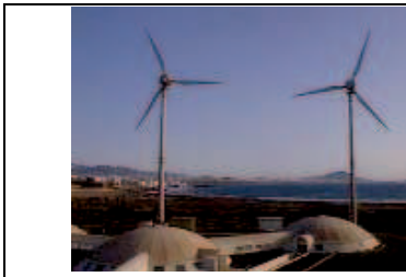
Figure 4. 2 x 225 kW off grid wind farm.
