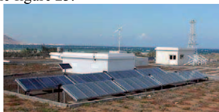
Figure 23. View of the solar collectors field coupled to the H/D desalination system.
