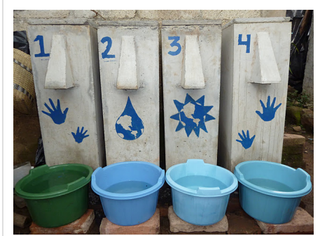
Biosand Filters implemented in Socorro, Guatemala by Engineers Without Borders from the University of Illinois: Urbana-Champaign
