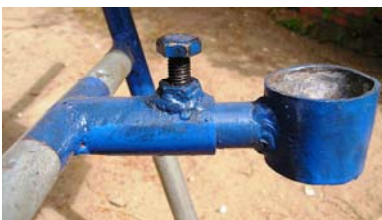
riser pipe support on structure
