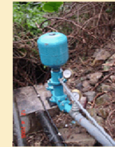
Pressure Vessel - serves as a buffer and catch up the over pressure
