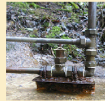
Delivery Pipe - pipe from the ram pump to a collection tank
