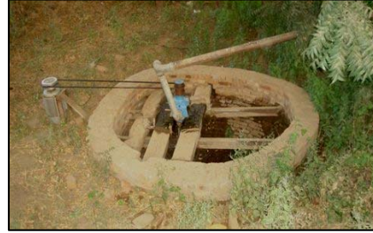
Pic 3: Electricity powered water pump.
