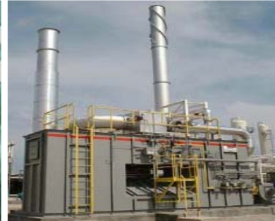
Paint Shop: Zero VOC Emission Regenerative Thermal Oxidizers [RTO] eliminate all VOCs in Exhausts
