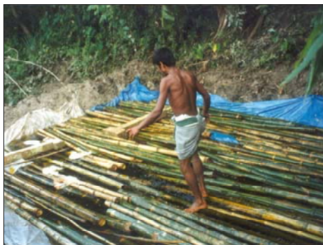
Figure 4: Curing bamboo trees for building Flood proof houses Faridpur, Bangladesh. Photo: Practical Action Bangladesh.
