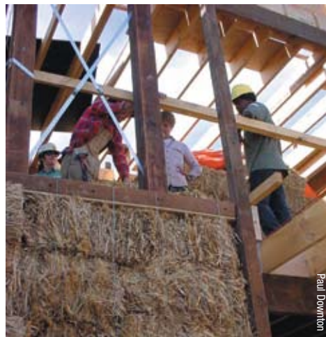
The middle plate and vertical compression wires can be seen in this detail of a timber framed three storey straw bale townhouse.
