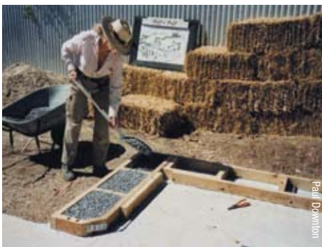
Ladder frame being filled with pea gravel prior to frame and bale placement.
